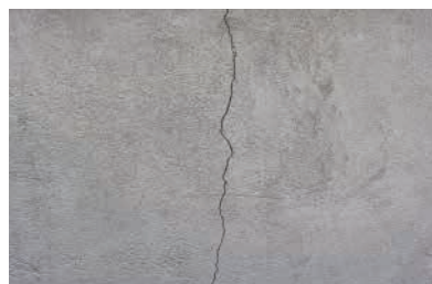
FIGURE G1.3.1.1(A): CRACKED CONCRETE
