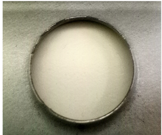
Rough, sharp edges of an inferior Steel Stud service hole
